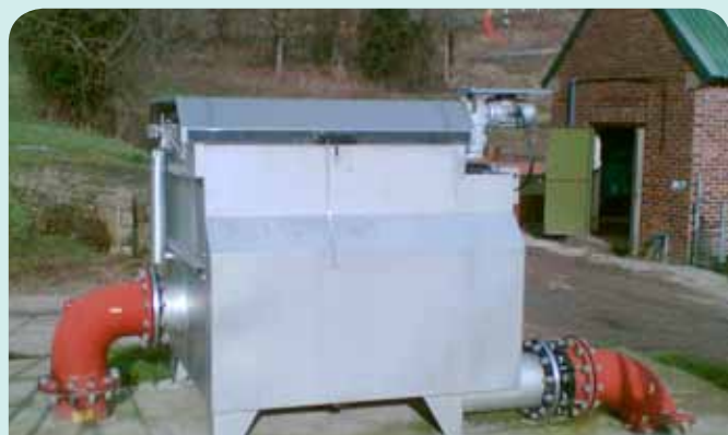
Site : Cuxton | Southern Water | 34 l/s site
